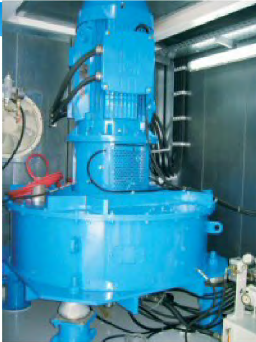
Flywheel energy storage. Source: Enercon.
