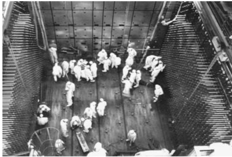
Figure 12. Assembly of the core of the C reactor at Hanford, state of Washington.
