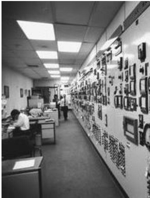
Figure 21. Reprocessing canyon F control room.
