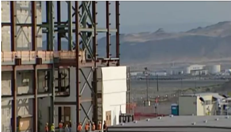
Figure 47. Waste treatment plant under construction at Hanford for the eventual glass vitrification of the waste.
