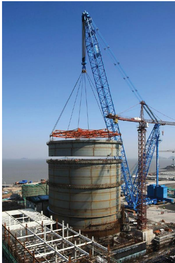
Figure 19. Toshiba-Westinghouse Next Generation first AP1000 reactor under construction since March 2009 at Sanmen 1, China by Shandong Nuclear Power Company. Reactor is slated for operation in 2013. Photo: Westinghouse Electric.
