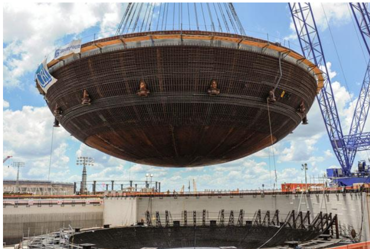
Figure 2. Georgia Power Vogtle 3 PWR unit 900 tons bottom of pressure vessel installation, Georgia, USA, 2013.
