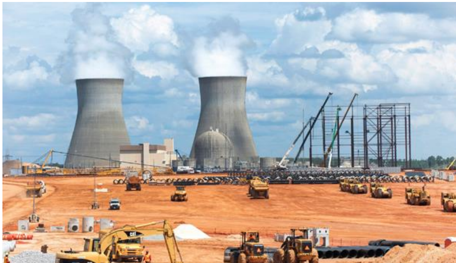
Figure 17. Active construction at the Vogtle units 3 and 4 reactors. Source: Southern Nuclear Company.
