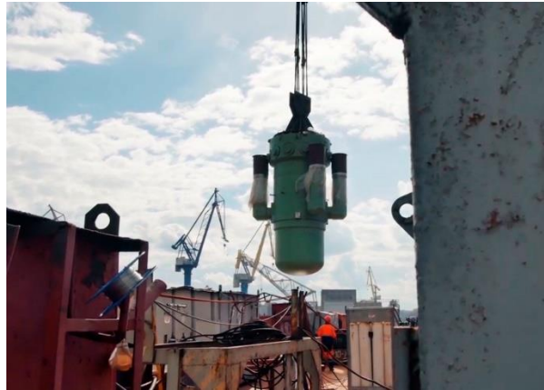
Figure 103. Pressure vessel of Russian icebreaker being installed. Steam is used for propulsion as well as jets to melt the ice.
