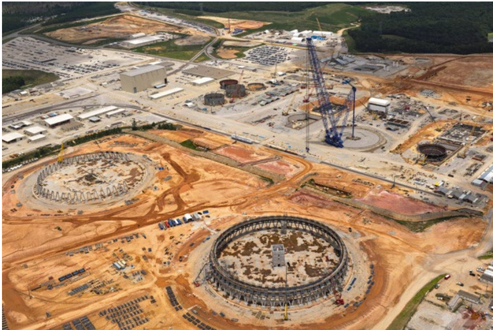
Figure 42. Georgia Power Vogtle plants units 3 and 4 under construction. Unit 3 entered operation in 2023
