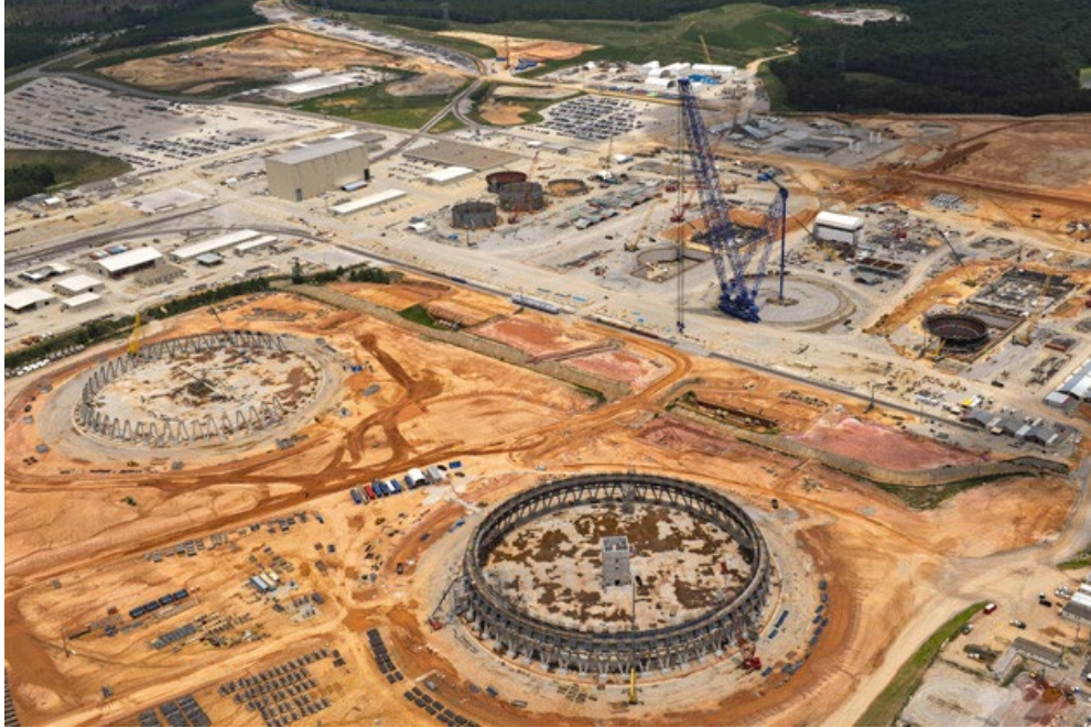
Figure 49. Georgia Power Vogtle plants units 3 and 4 under construction. Unit 3 entered operation in 2023 and unit 4 in 2024.
