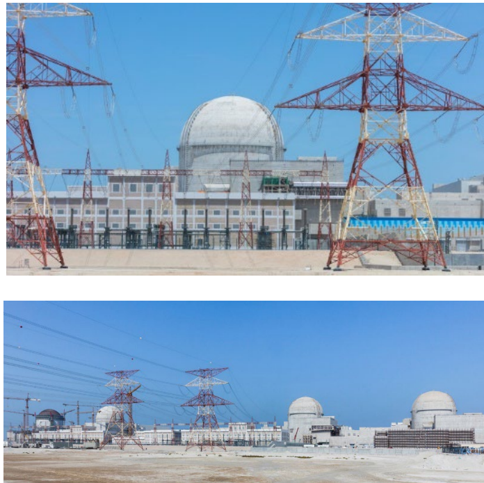
Figure 23. The Barakah four-unit South-Korean-designed APR-1400 reactors are being built at Barakah, in the Dhafrah region of Abu Dhabi, United Arab Emirates (UAE) by a consortium led by Korean Electric Power Corporation (Kepco). Construction began on the first unit in July 2012, unit 2 in May 2013, unit 3 in September 2014 and unit 4 in September 2015. The Barakah plant was developed by the Emirates Nuclear Energy Corporation (ENEC). The 1,400 MWe Unit 1 started operation in August 2020. The four units are expected to supply 25 percent of the UAE's electricity demand.
