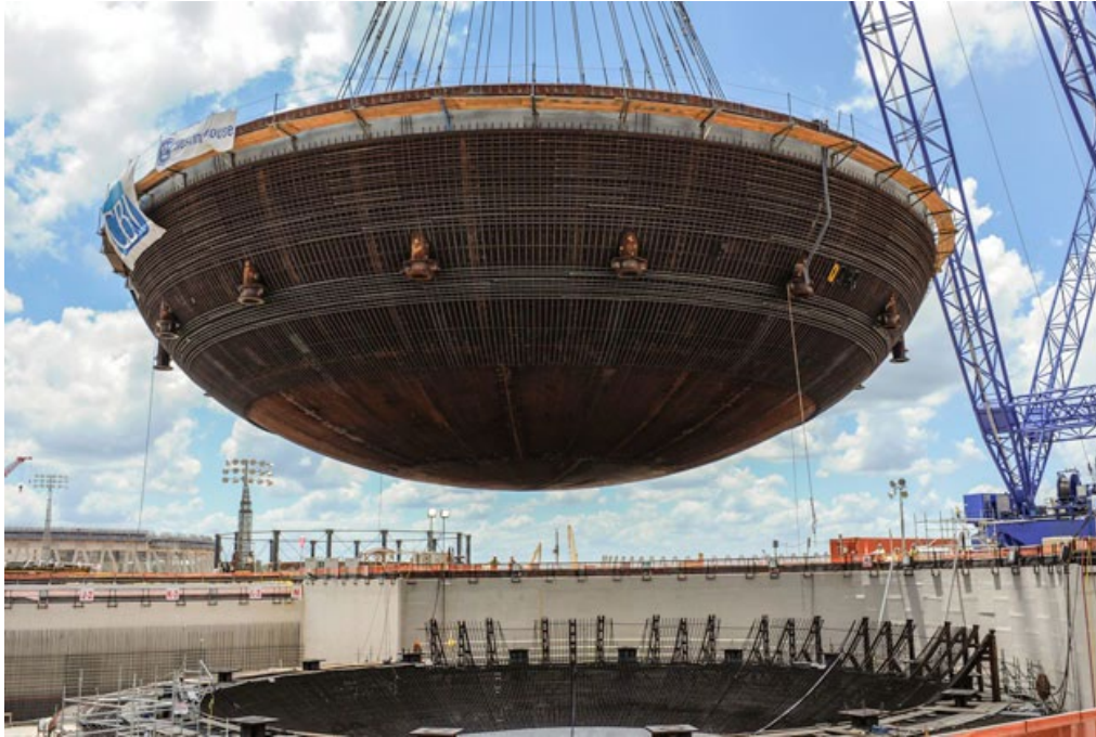
Figure 43. Georgia Power Vogtle 3 PWR unit 900 tons bottom of pressure vessel installation, Georgia, USA.
