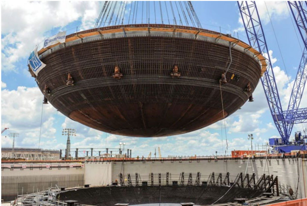
Figure 50. Georgia Power Vogtle 3 PWR unit 900 tons bottom of pressure vessel installation, Georgia, USA.
