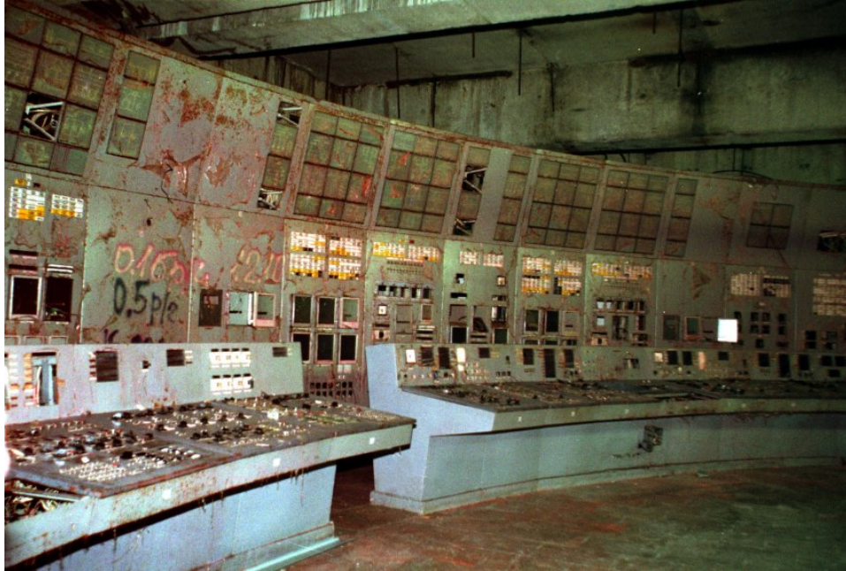
Figure 16. Remnant of Control room of Chernobyl unit 4.
