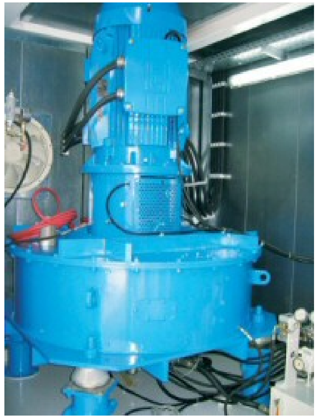
Figure 7. Enercon Flywheel. Source: Enercon.
