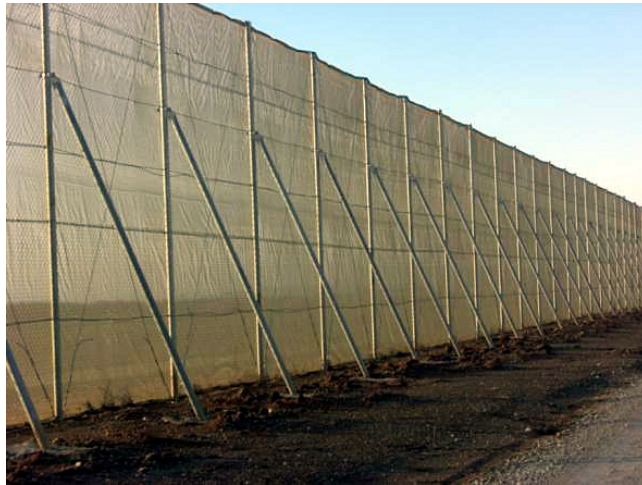
Figure 2, Protective walls to protect structures against wind loading at Al Kuraymat, Egypt [16].
