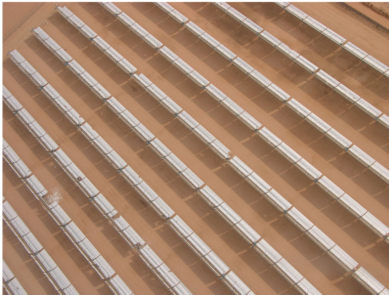
Figure 1. Trough reflector system showing damaged mirrors needing replacement.
