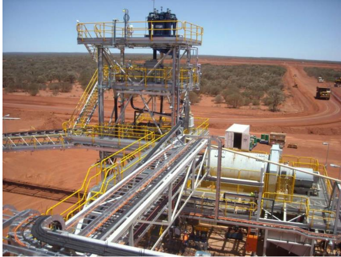
Figure 29. Ball mill and classification circuit at concentration plant. Source: Lynas.
