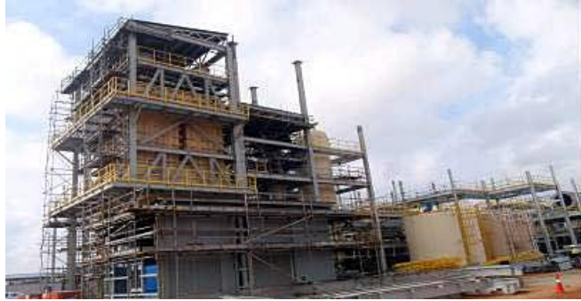
Figure 46. Gas treatment plant.
