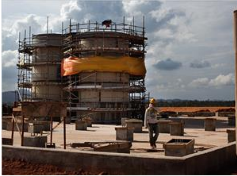
Figure 43. Rare earths refinery tanks.
