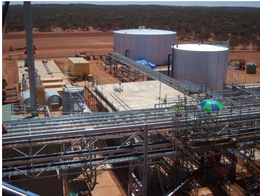
Figure 30. Utilities concentration plant.
