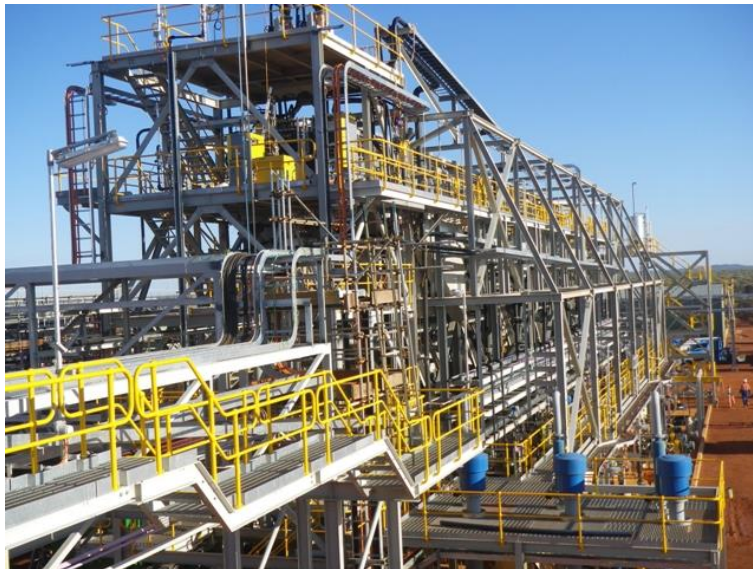
Figure 28. Flotation section at the Concentration plant at Mount Weld, Australia. Source: Lynas Corporation.
