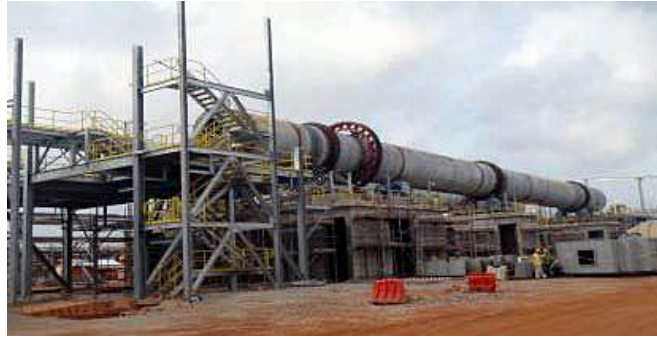
Figure 40. Cracking rotary kiln at processing plant. Source: Lynas.
