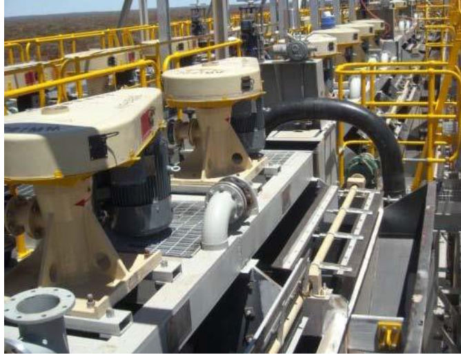
Figure 31. Flotation cells at concentration plant.
