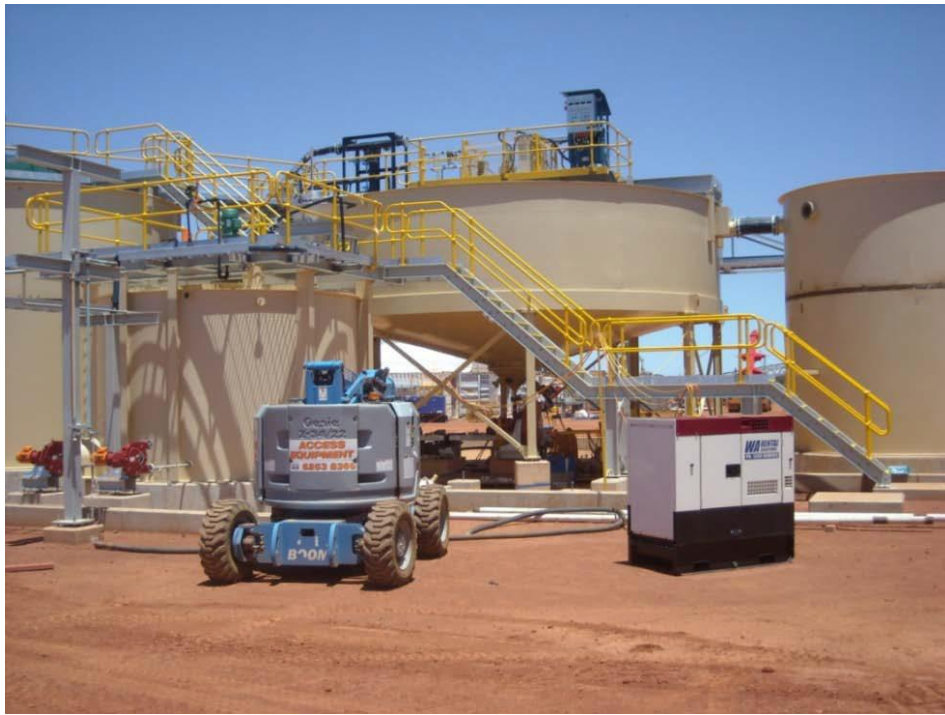
Figure 36. Thickener concentration plant.
